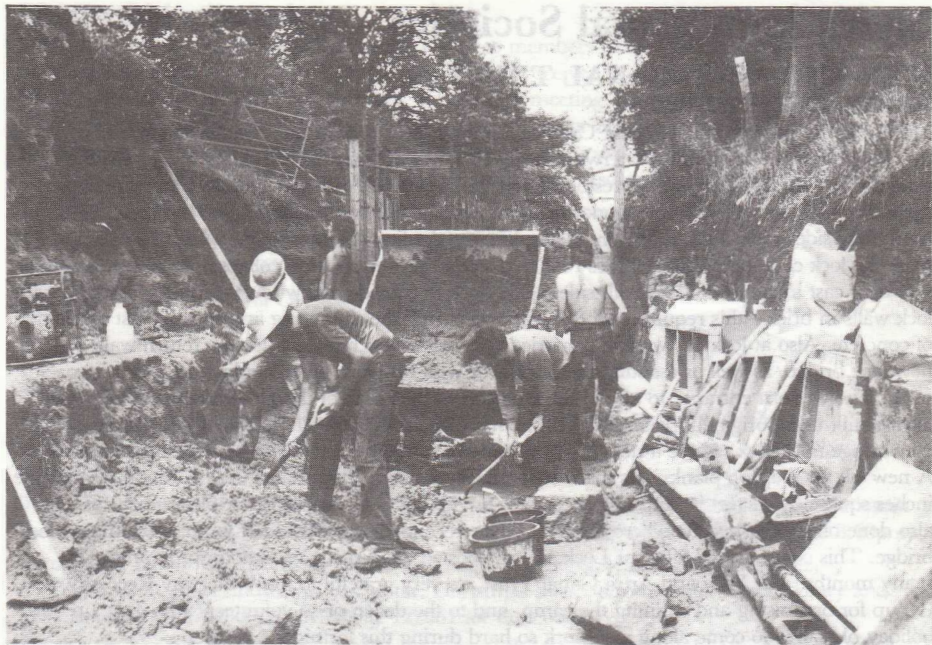
Members of the Waterway Recovery Group at Lock 17, Wey and Arun Canal—July 1983
